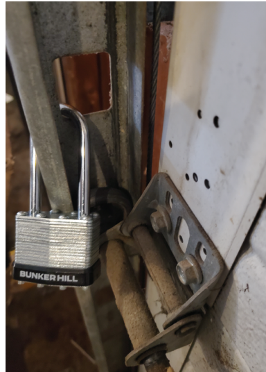
Padlock on garage door.
